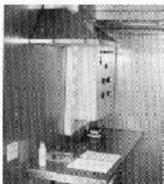
Workplace with air cleansing system
